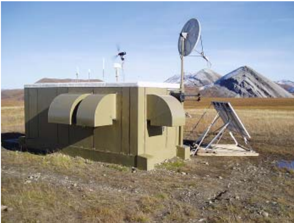
The power module at Ivotuk, Alaska, after installation of PV and wind.
