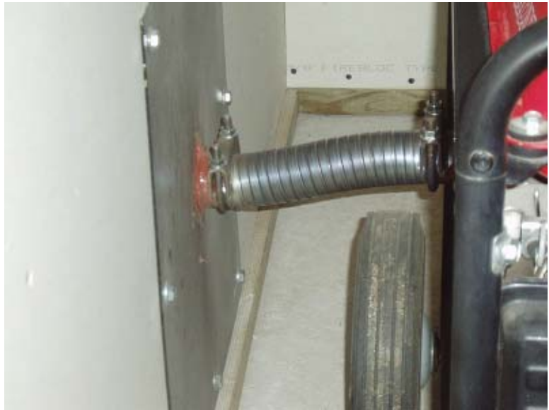
Combustion exhaust gases are poisonous and very hot (>500F). Penetrations in enclosures must be properly designed for safety and reliability. Note the large flange and flexible, high-temperature connector pipe.
