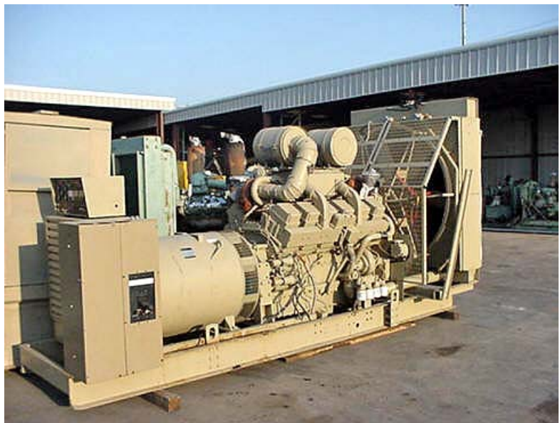
The Cummins 800kW generator.
