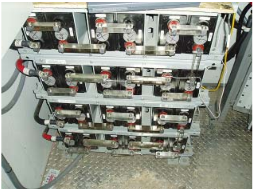
Industrial battery stacks offer the ability to reconfigure voltages based on 2 volt cells. They can also allow for a lot of energy storage in a compact space.
