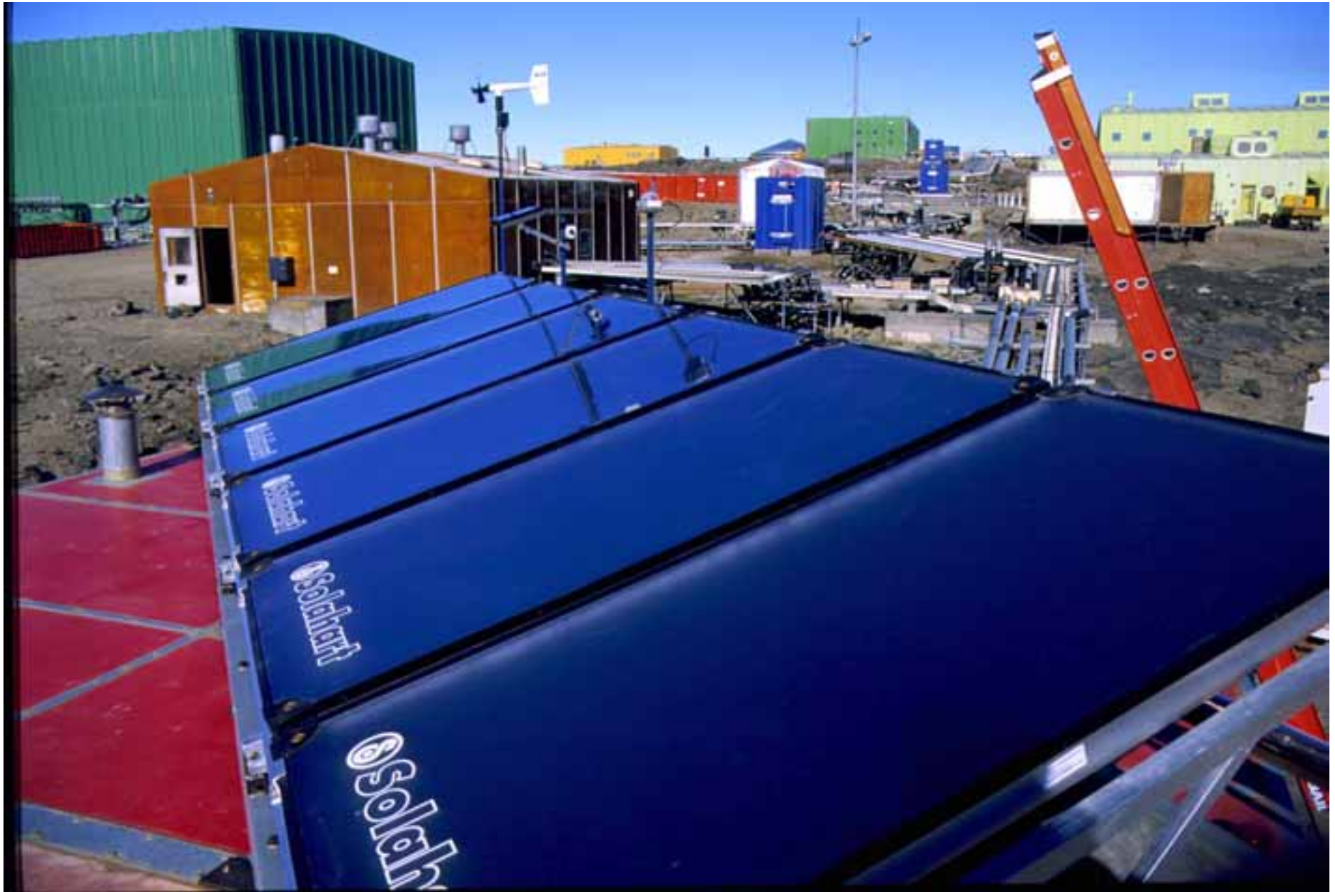
Pilot Solar Hot Water System, Davis Station, Antarctica, 1998/1999
