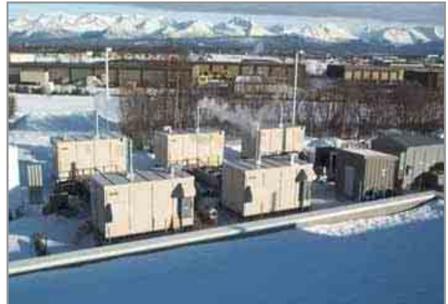
Chugach EA's 1000kW Installation at Anchorage Post Office
