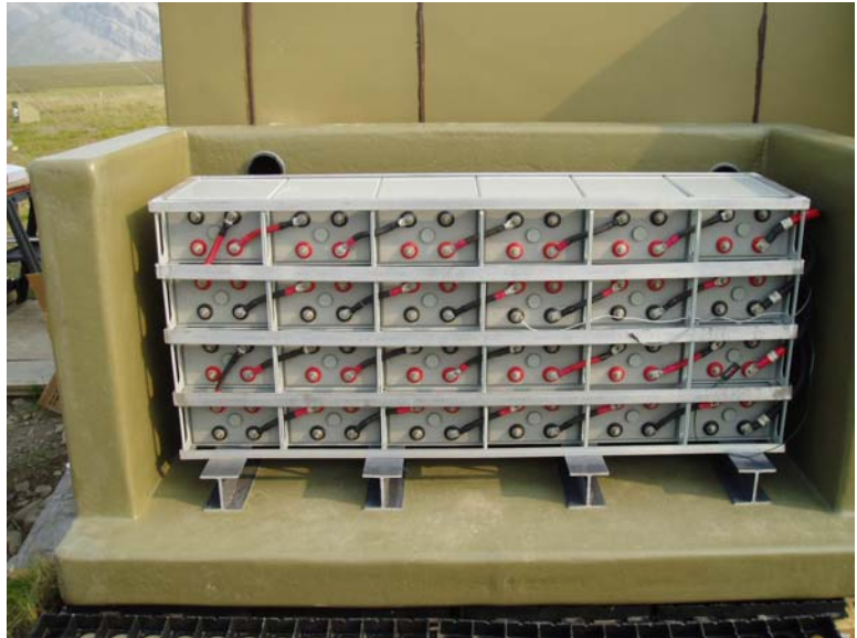
Industrial battery stacks offer the ability to reconfigure voltages based on 2-volt cells. They can also allow for a lot of energy storage in a compact space.
